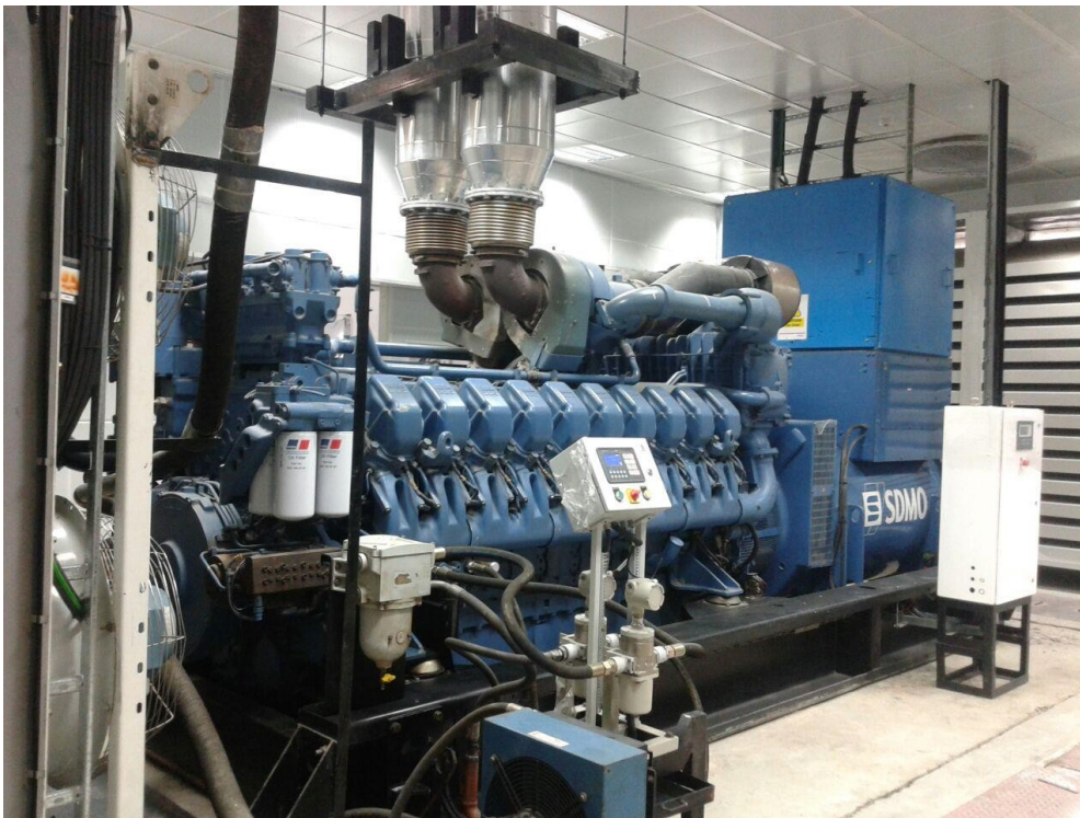
Fig. Installation of FCM on 3000 kVA MTU Engine, Infosys Chennai Campus
