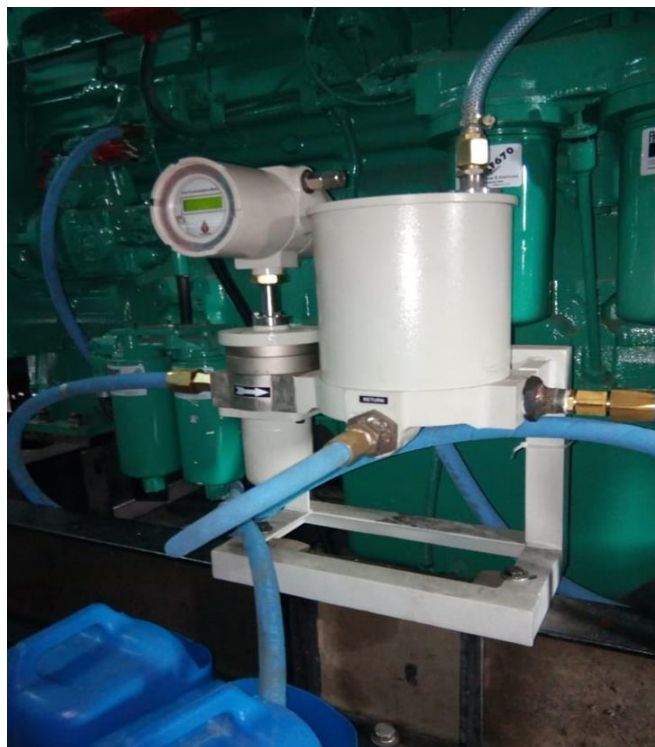
Fig. Installation of FCM on 500 kVA Cummins PT Based Engine, Railway Power Car
