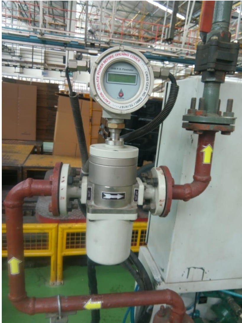
Fig. Positive Displacement Flow meter used to measure inline flow
